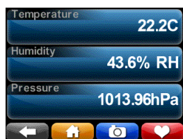
PQube3 screen of ambient conditions at a data center
